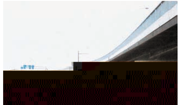
Photo 5 Appearance of World-cup-kyo Bridge applied with CUPTEN COAT M treatment and pre-coat system (Yokohama City)
